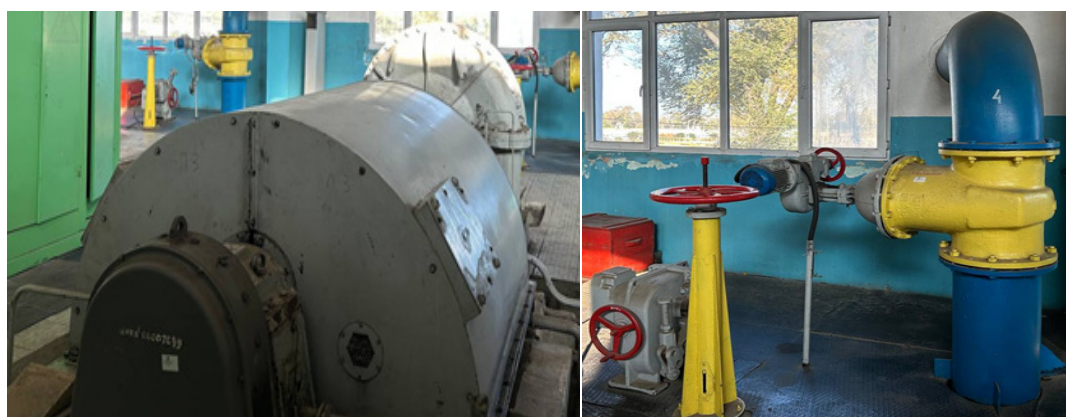
Figure 2 – Supercharger and the outlet pipe of the blowers of the aeration station, Almaty city
